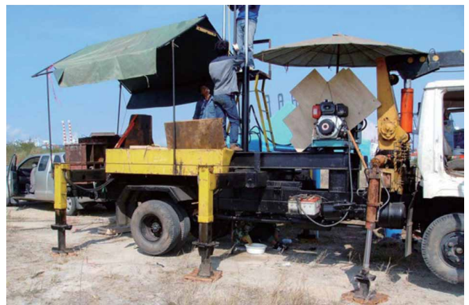
Nong Saeng Natural Gas Power Project, Thailand
