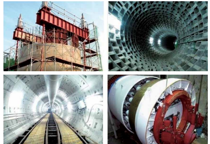
161KV Cable Transmission Links (Anan to Fucheng) and Underground Section from Anan to Yun River
